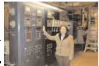
Lorinda Gussow explains the dual-fuel boiler control system at Rockland Community College.
