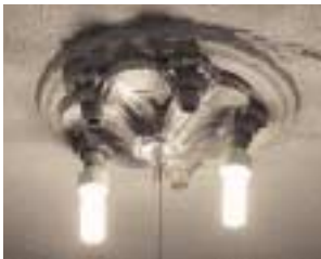
Compact fluorescent bulbs installed to replace incandescent lighting.
